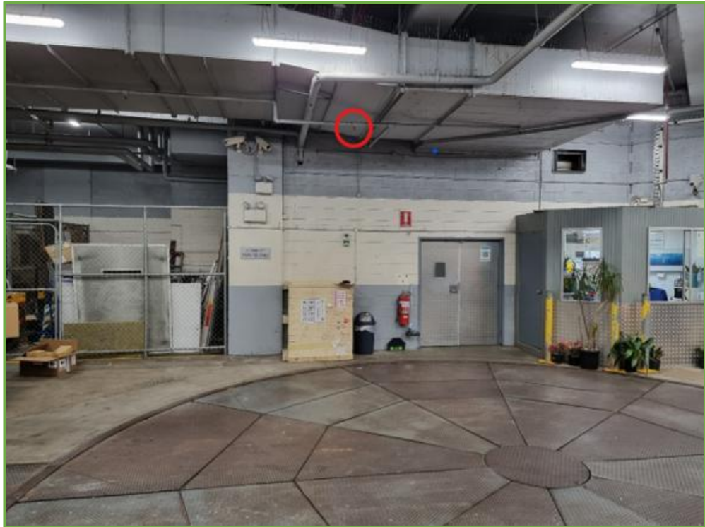
Figure 1: 3.5m Clearance Measured from Turntable to Overhead Sprinkler as Circled in Red Above
